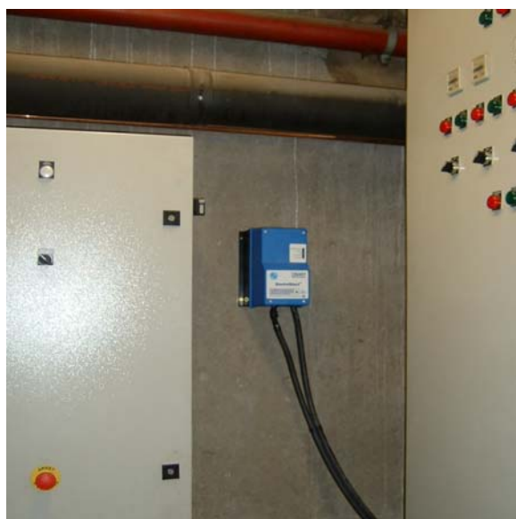
Mounting of EnviroStart adjacent to Control Panel
