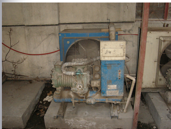
The Refrigeration Compressor Pack on Which the Testing was Conducted.
