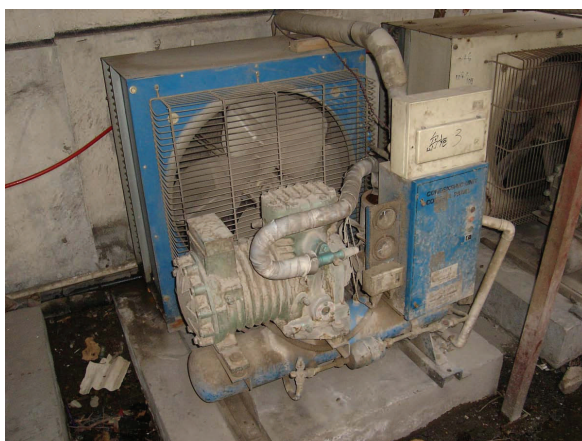
The Chiller on Which the Test was Conducted
